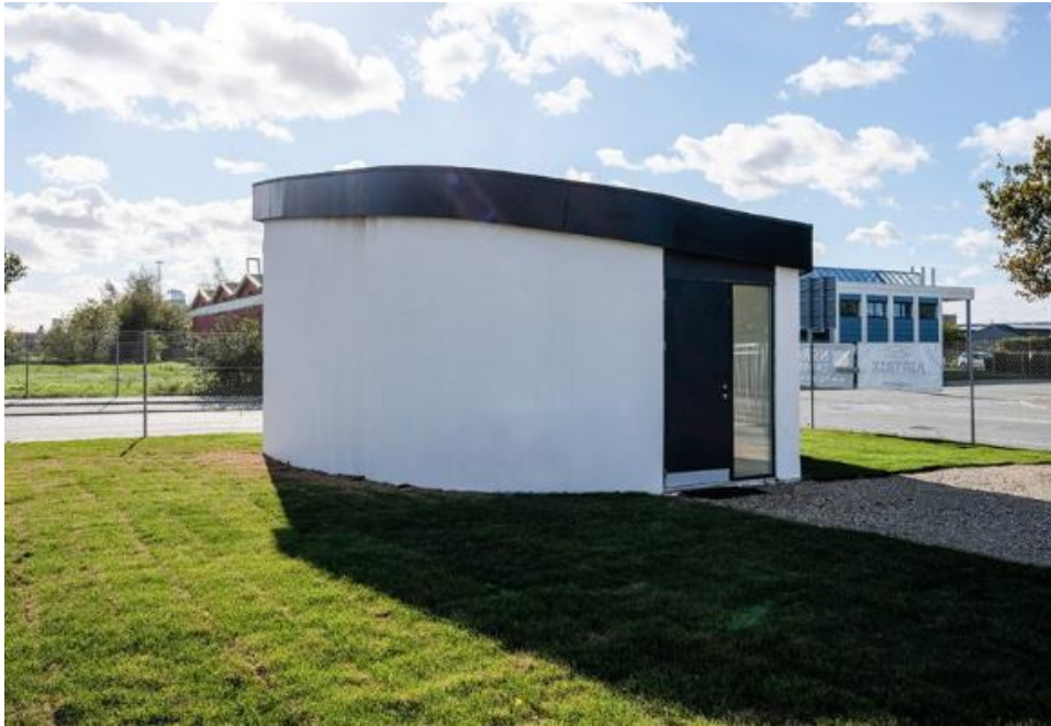
Figure SI17. Picture of the house 3D-printed in Denmark by COBOD. Retrieved from Case stampate in 3D: Cobod - 3D 4Growth .
